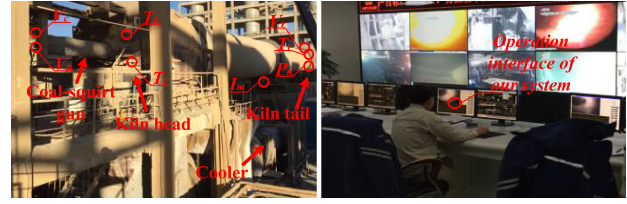
Fig. 11. Installation locations of sensors (left) and the central control room (right).
